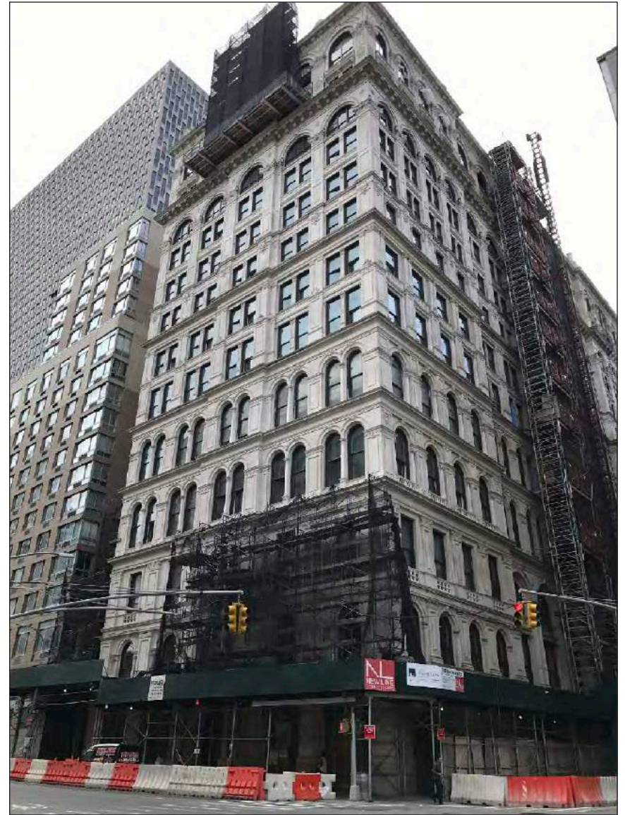
The New York Life Insurance building with frontages on Lafayette Street and Broadway 22
