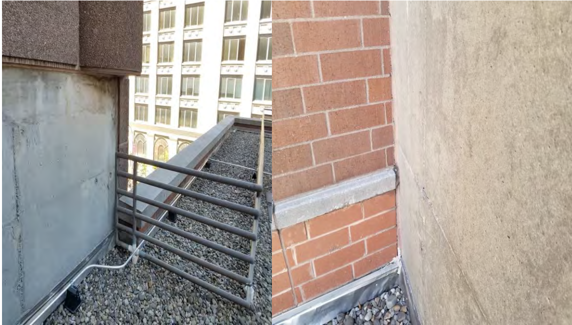
Overhang Encroachment, and butt joint without separation.
