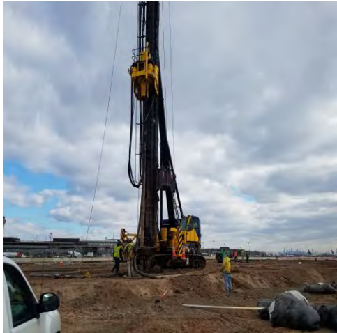
Pile drilling rig at Newark Airport. A rig of this size is necessary to drill to sufficient depth for the jail site. (authors
